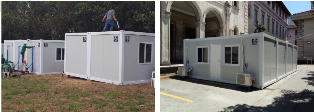
With member firms and those of its affiliate, PSVARE, assisted EEI Corporation to quickly set up 60 emergency medical facilities used by eight hospitals in the cities of San Juan, Mandaluyong, Manila, and Quezon, as well as in Antipolo City in Rizal, Santa Rosa City in Laguna, and Batac City in Ilocos Norte
